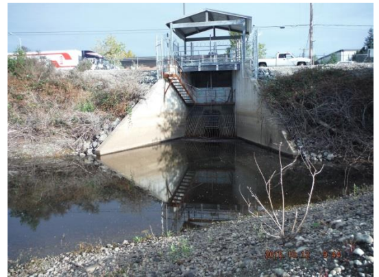
Gravel Pit Stormwater Regional Facility and Outlet Structure
